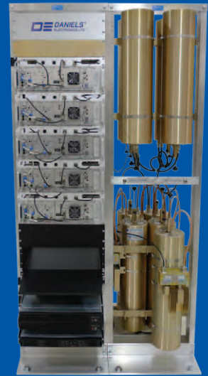
P25 Trunked System
