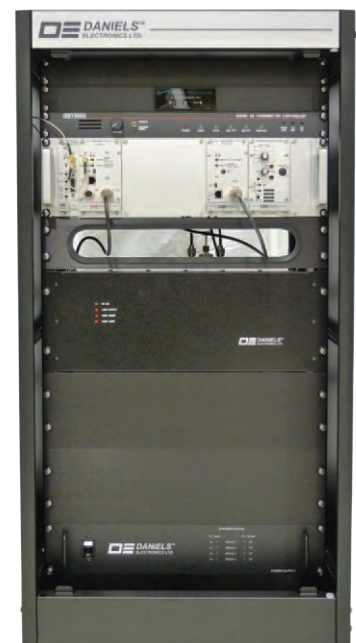
Paging Transmitter with 100 Watt Power Amp
